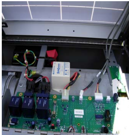
The control panel and battery under the solar panel.
