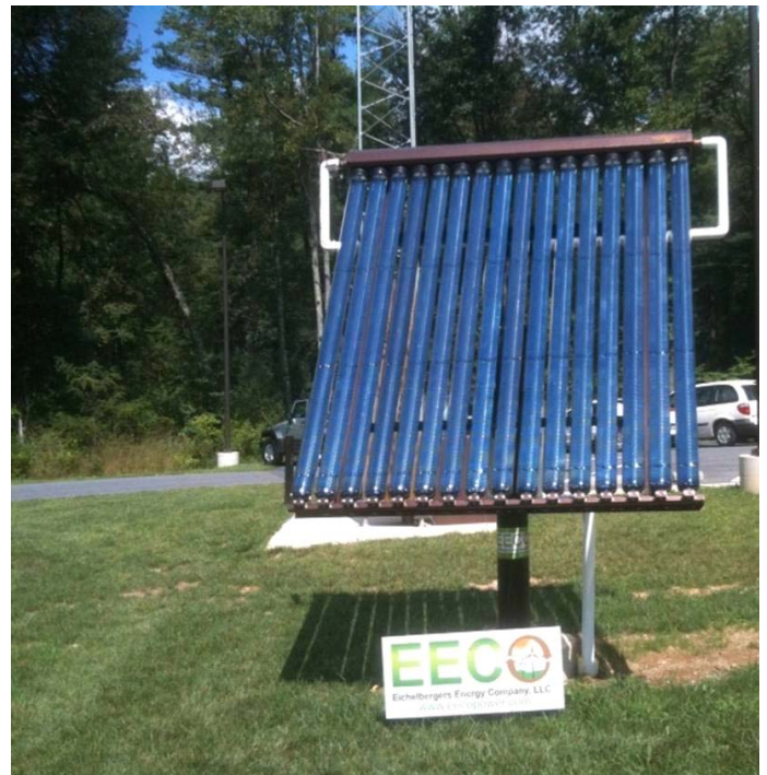
A thermal (Evacuated Tube Array) panel was recently installed at Caledonia State Park. It is creating hot water for the Park’s Office.
